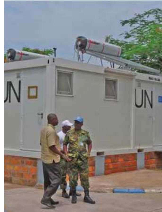
Solar water heaters are mounted on the roofs of sanitary units at a UN peacekeeping base in Kinshasa, DRC
