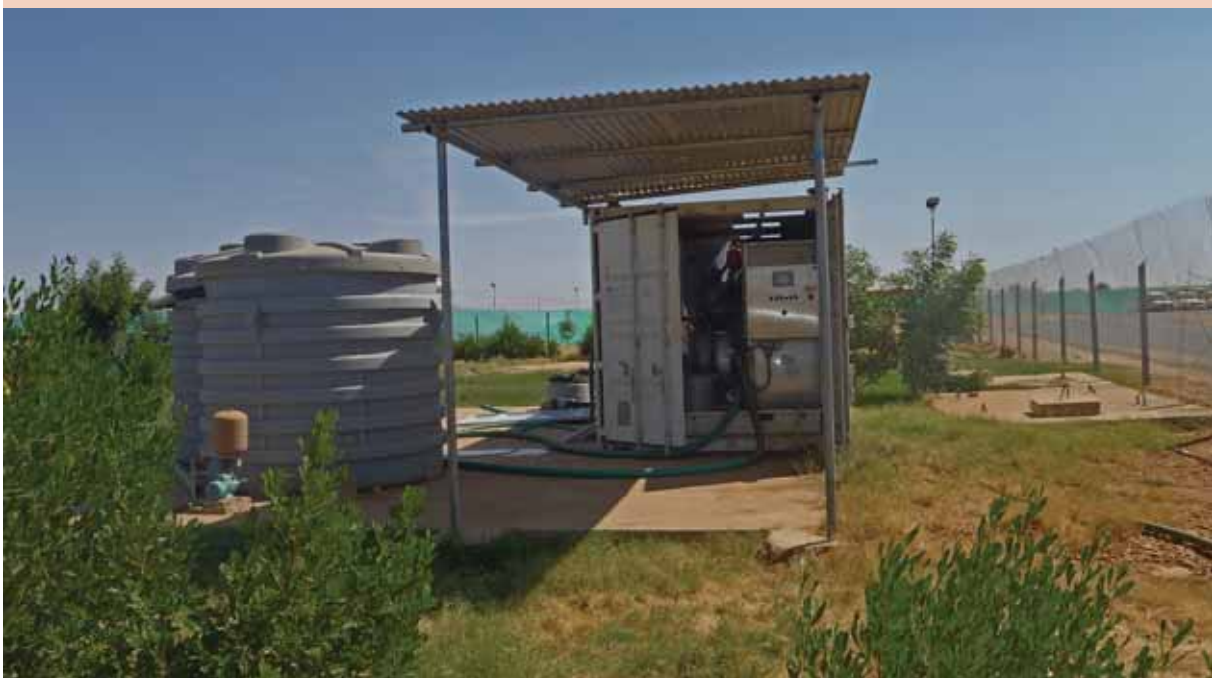
Wastewater treatment plant, El Fasher, Darfur
