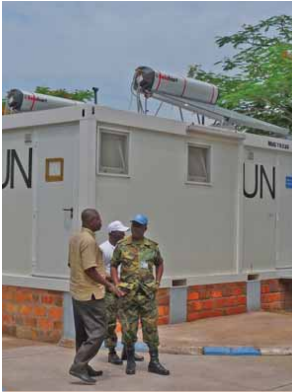
Solar water heaters are mounted on the roofs of sanitary units at a UN peacekeeping base in Kinshasa, DRC
