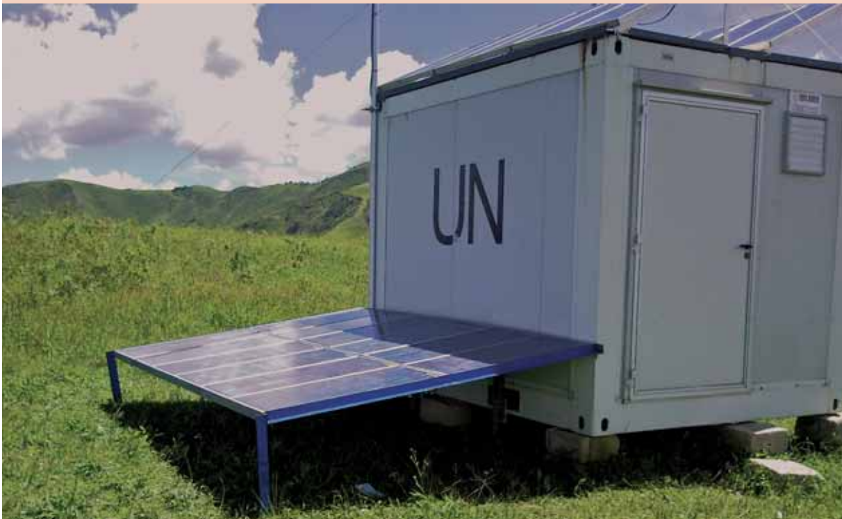
The peacekeeping operation in Timor-Leste powers remote VHF (very high frequency) repeaters with solar panels
